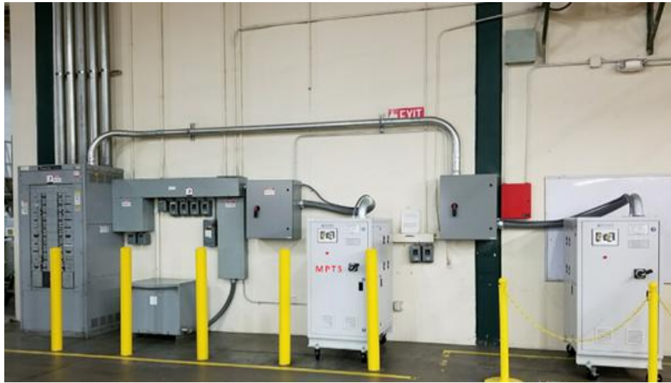
Figure 7. Citrus packaging plant using two PMCS units
